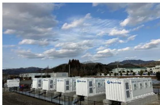
Storage power plants: 1,999 kW-6,000 kWh
