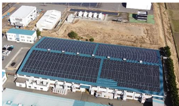
Solar power generation facilities: Approx.1,000 kW High-voltage consumer: Japan Power Fastening Co., Ltd.
